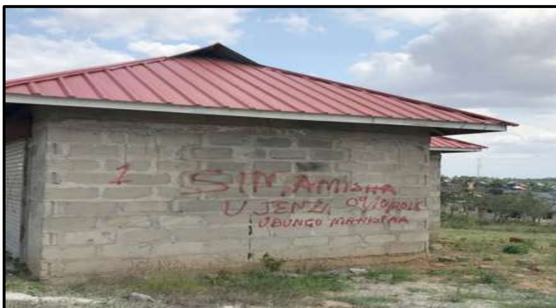
Plate 4. 6 Stop order on ongoing construction at resettlement area
