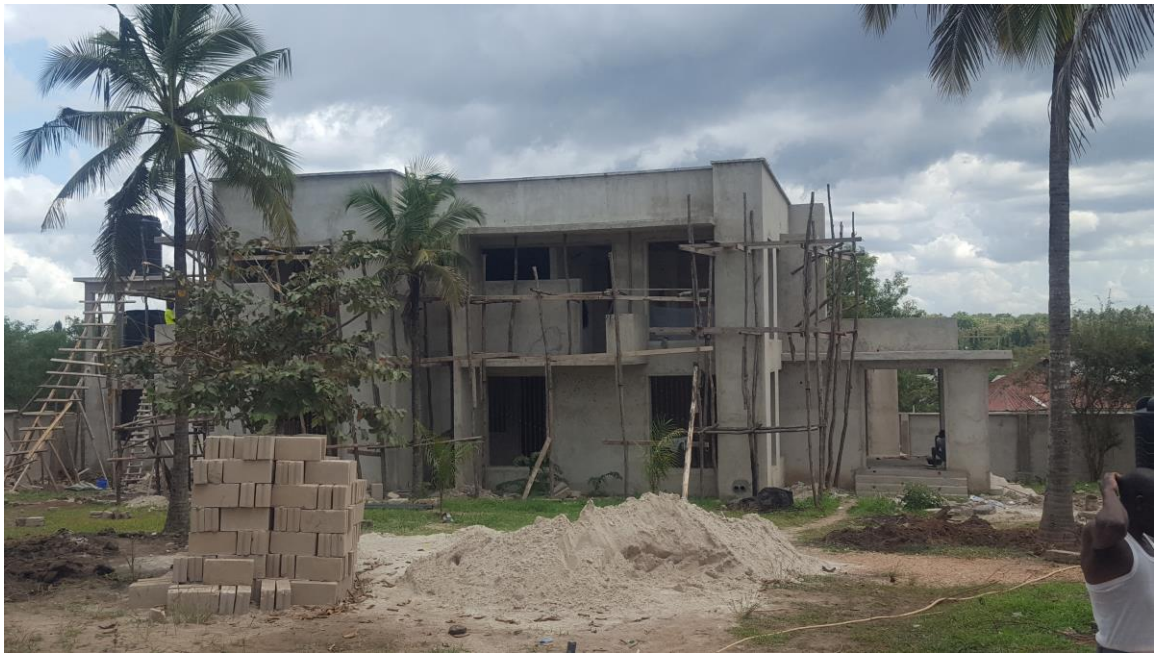
Figure 4.2: Construction of Double Storey Residential House at Finishing Stage; the Developer did not Register the Project to any Regulatory Board
