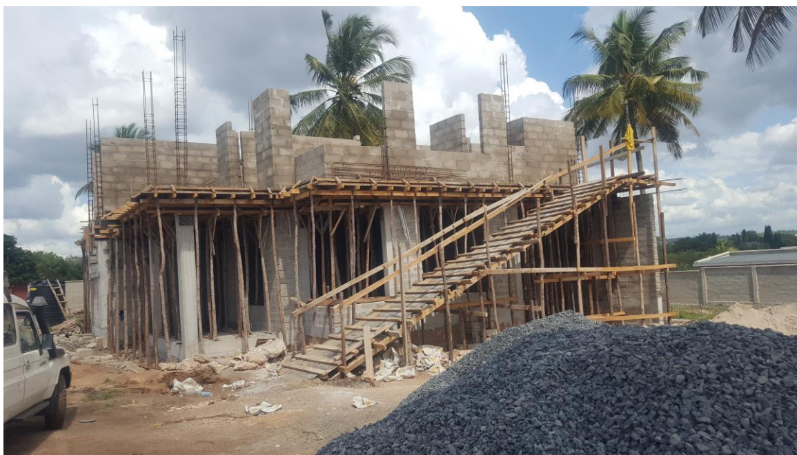
Figure 4.1: Construction of Double Storey Residential House at Block Work Stage; the Developer did not Register the Project to any Regulatory Board.
