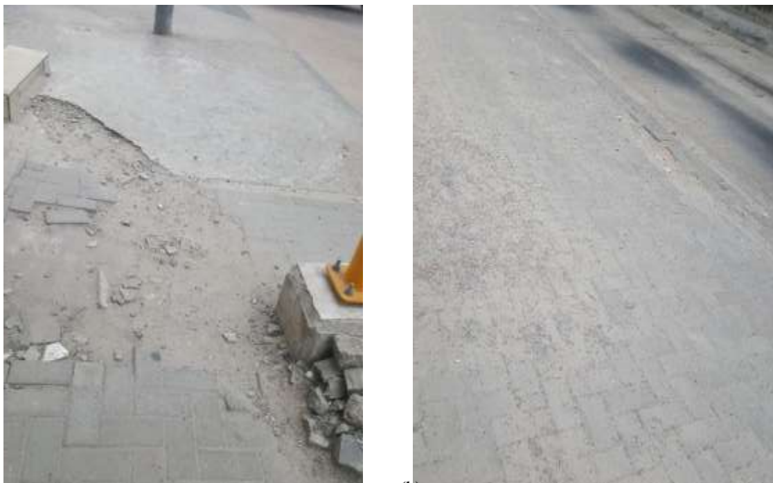
Figure 4.8: (a) and (b) untimely response to defects increases the magnitude of defects on road shoulders
