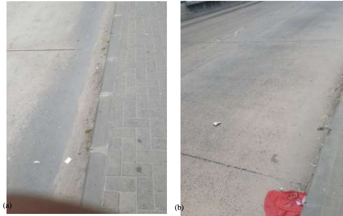
Figure 4.7: (a) and (b) the uncleansed road surface caused by informal wastes management and vendors' activities taking place along the BRT road infrastructure
