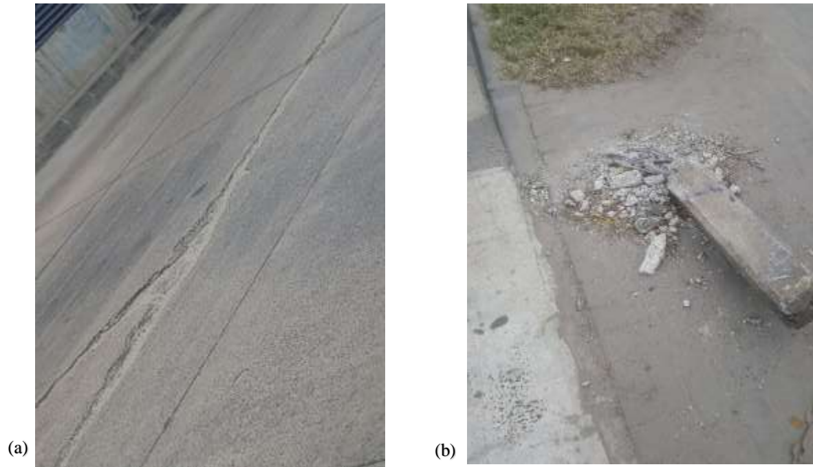
Figure 4.3: (a) multiple cracks, (b) damaged bollards in BRT road
