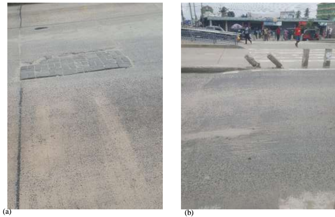
Figure 4.4: (a) Concrete road patch repaired with sand cement pavers, (b) damaged bollards and un-painted zebra crossing (markers) in BRT road.
